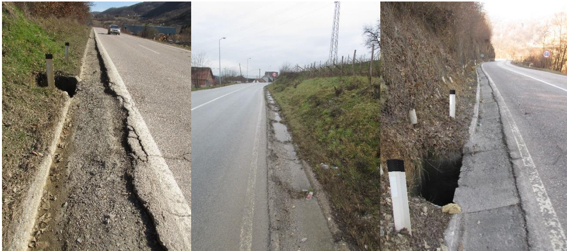
Figure 12. The gutter on the observed road section
